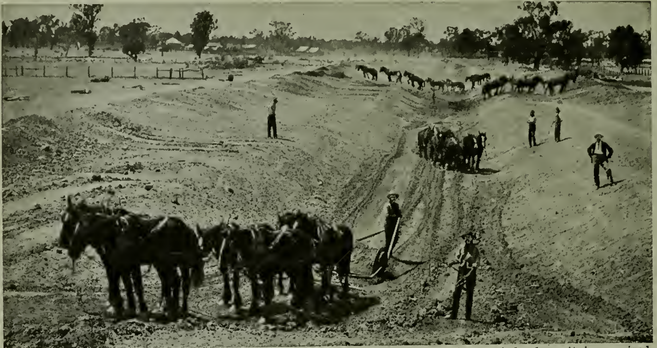
A great dam is only one part of an irrigation scheme. The water must be carried where it is required. The channel of the Murrumbidgee irrigation scheme in Australia, 138 miles long, is being hollowed out.
